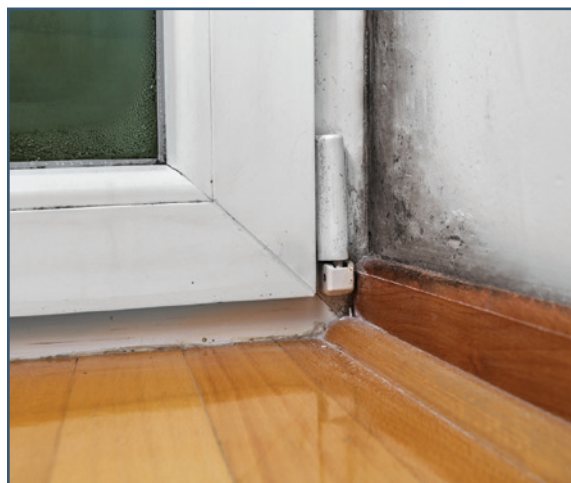
Mold in residential building
